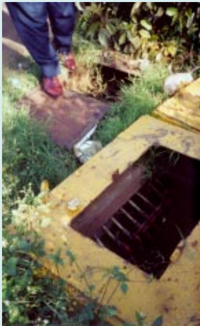
A metered manifold box.
