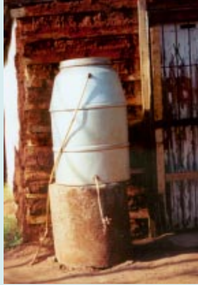
A semi-pressure system with a ground tank.
