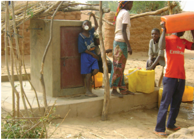
A stand pipe for water supply in the region of Tahoua, Niger (Photo: Taibou Adamou Maiga)
