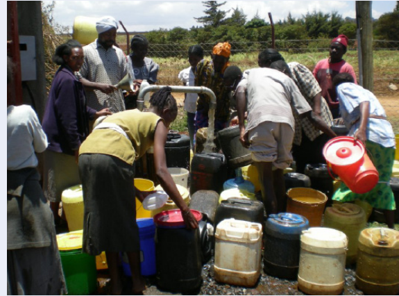
Community water point at Gitaru Water Project in Kiambu district, Kenya. Gitaru received a loan of $60,000 to equip a new borehole and install distribution tanks in the project area. As a result, residents now have a constant water supply and the project has been able to expand the number of connections it supplies by 20%.
