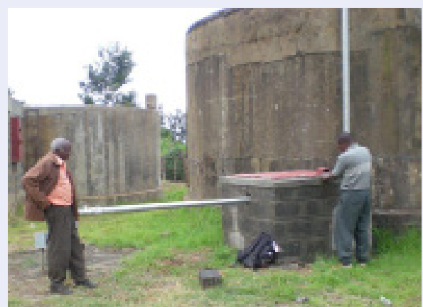
Storage and distribution tanks at Karaweti Water Project in Githunguri division of Kiambu district. The community borrowed $50,000 from K-Rep Bank to develop a new source and install meters for all its customers. As a result, revenue collection increased by 90% and the reliability of water services increased tremendously, with 87 percent of customers receiving water seven days a week, up from 8 percent before the investment.
