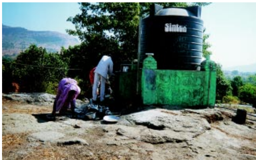
A storage tank and public standpost in Hadshi, Pune.
