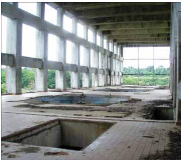
The hydro plant at Mt Coffee was completely looted during the war. The round holes are where the pumps used to be.
