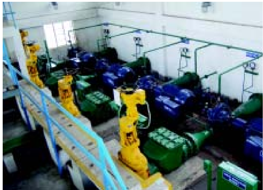
Booster pumps at the water works.
